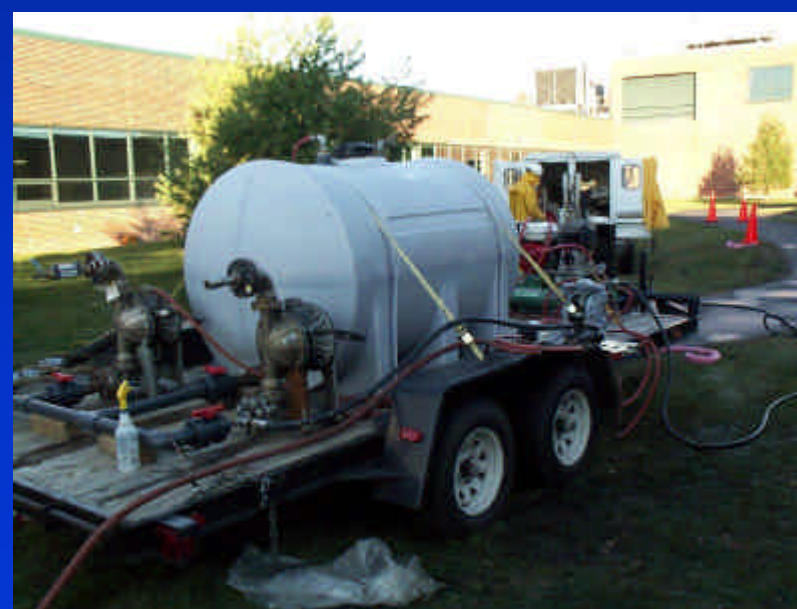
Trailer-mounted pumping system used to pump permanganate from tanker truck into injection points
